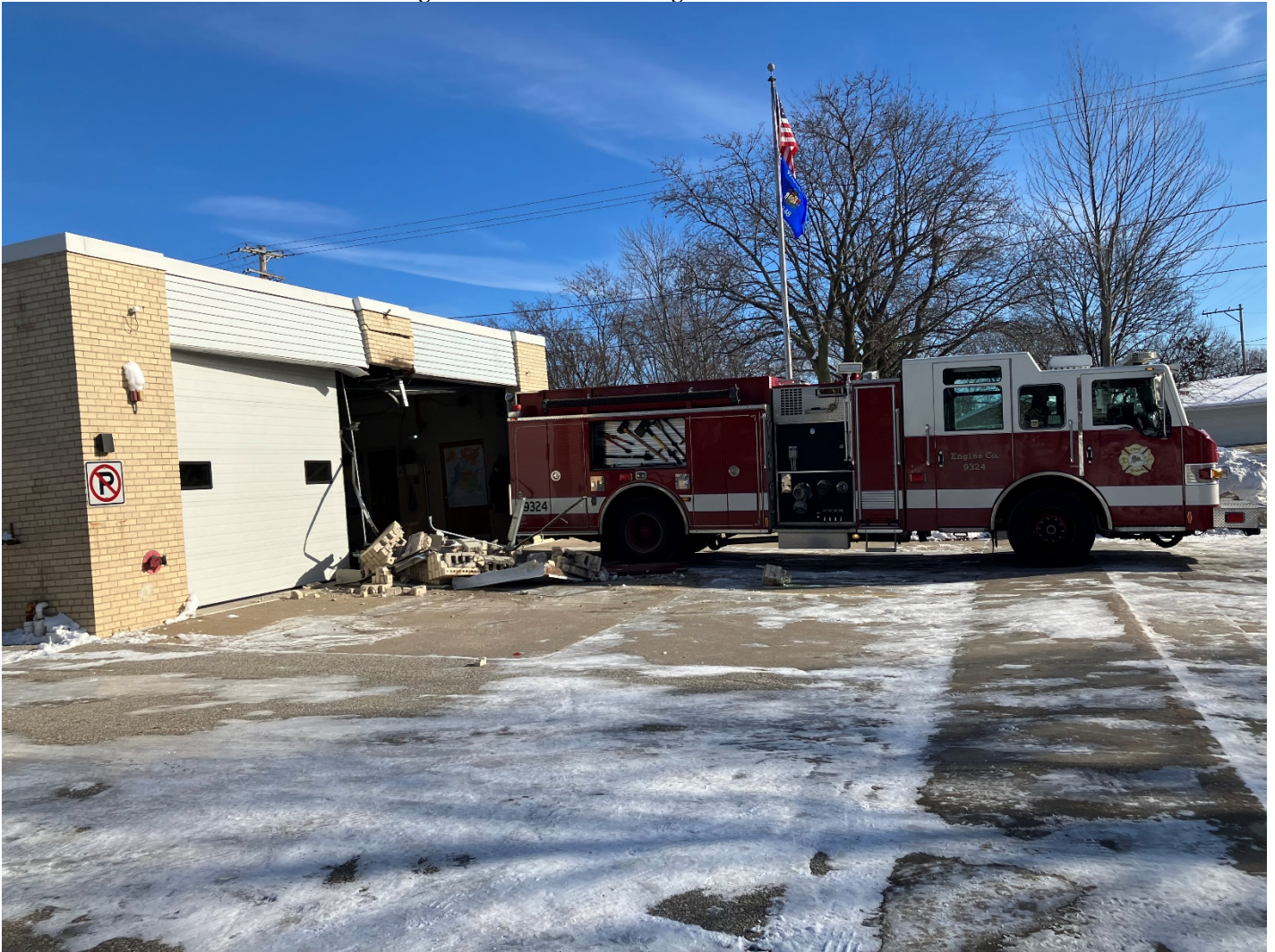
Figure 3: Fire Station #4 rig struck exterior wall.
