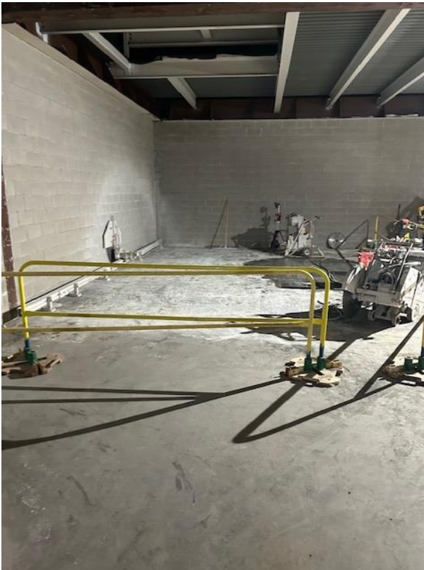
Freight Elevator – Upper Level
