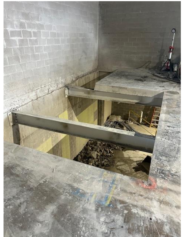
Freight Elevator – Upper Level
