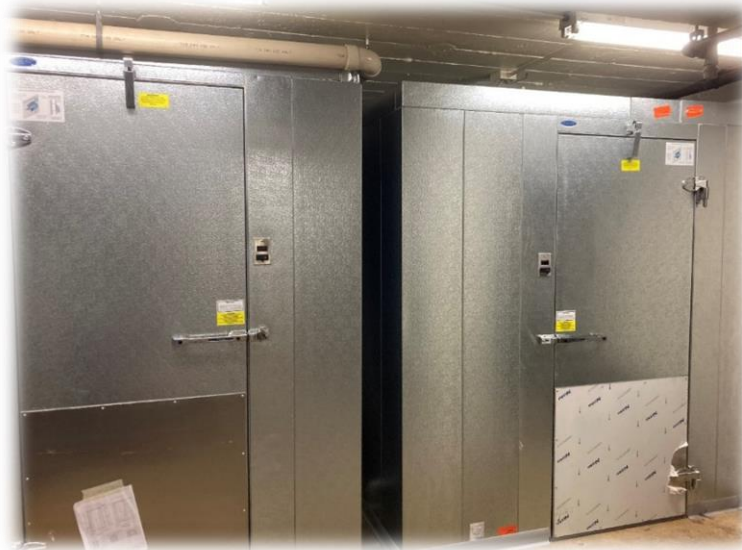
Clubhouse basement Freezer (left) and cooler (right).
