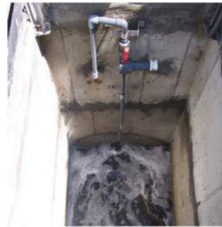
Enhanced Wet Detention (Coagulant Addition)
